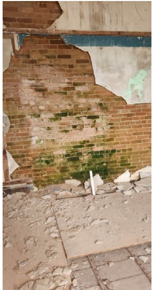
WALL COVERINGS Wall coverings have reached the end of their useful life and need to be replaced.
