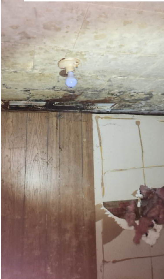
HOLES IN WALL CAVITIES Holes in walls cavities allow for water/rodent intrusion.
