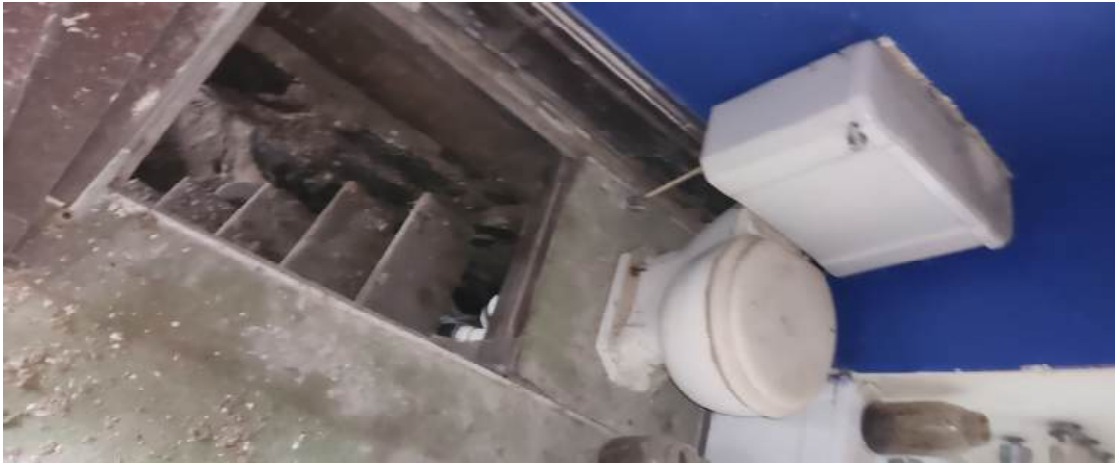
FUNGAL GROWTH Saturated wall coverings – fungal growth.
